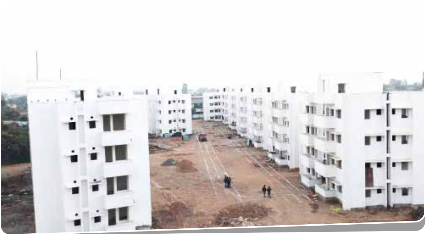
Client : Regional Institute of Medical Sciences | Total Area : 2,40,000 sqft | Location : Lamphel Road, Imphal, Manipur
